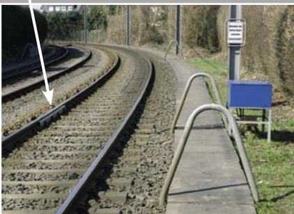
Rail head wetting on inner rails
